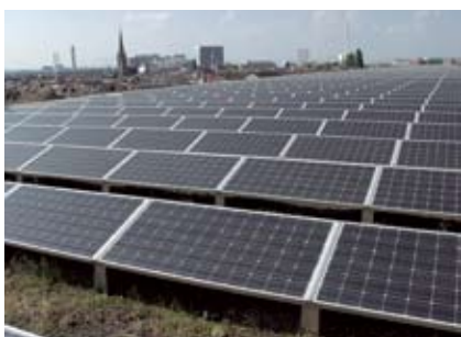
Photovoltaic panels on exposition building, Basel
