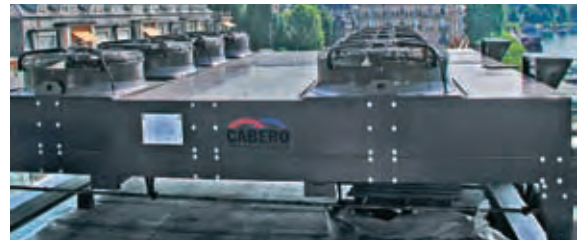
Colour-coordinated recooling unit on roof
