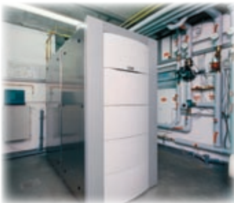
Photo: Vaillant GmbH fuel cell heater in a field test under normal working conditions
