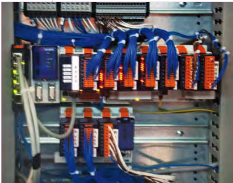
Pumping station control cabinet with Saia®PCD3 controllers
