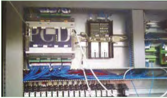
View into the cabinet of the new machine: Saia®PCD2.M5540 with Profibus connection.
